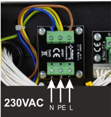
PCB Power Board im Patch Panel
