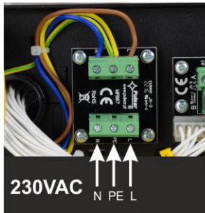
PCB Power Board in the Patch Panel
